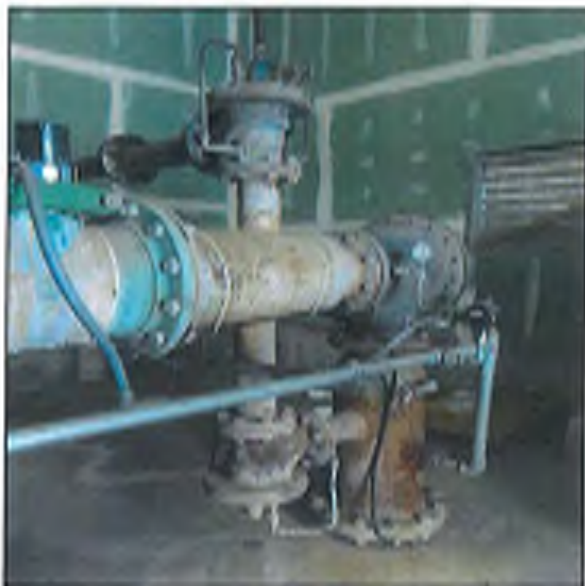
Fig. 9 – well # 7 sample tap, pressure gauge and pressure release
