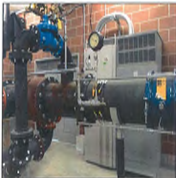
Fig. 67 – well # 11 sample tap and pressure gauge
