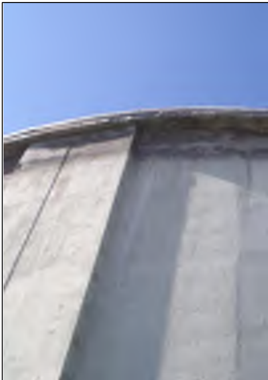
Exterior pilaster and underside of roof overhang, minor scaling at roof
