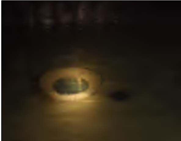
Tank outlet and drain, sand build-up at floor
