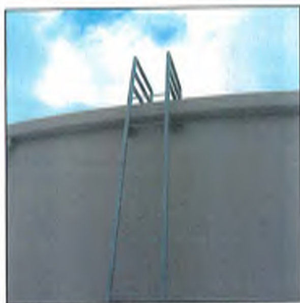
Fig. 17 – storage tank access ladder
