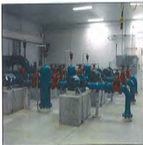
Fig. 51 – over view of booster station located below storage tank
