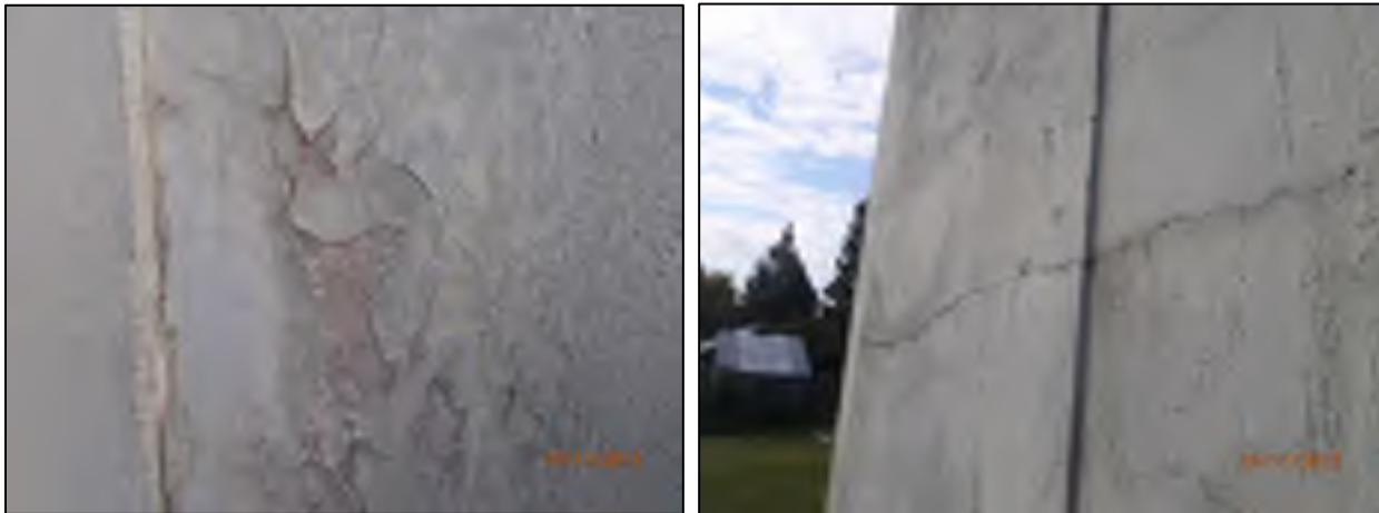
Surface scaling and cracking occurring in sack finish and coating
