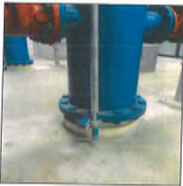
Fig. 53 – unscreened pressure release
