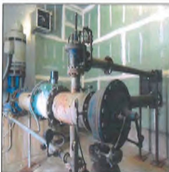
Fig. 13 – well # 7 check valve and overview of discharge line
