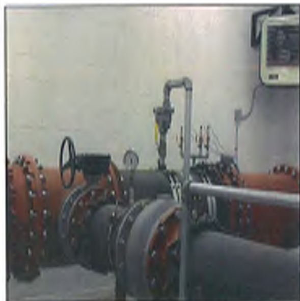
Fig. 28 – isolation valve, pressure gauge, pressure relief valve and pressure controller on discharge line from storage
