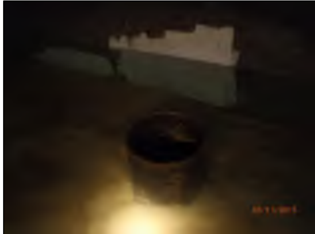
Tank inlet, up to four inches of sand at floor around inlet
