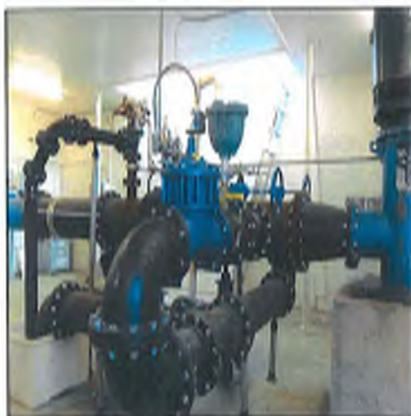
Fig. 44 – discharge piping of well # 10 (check valve and air release)
