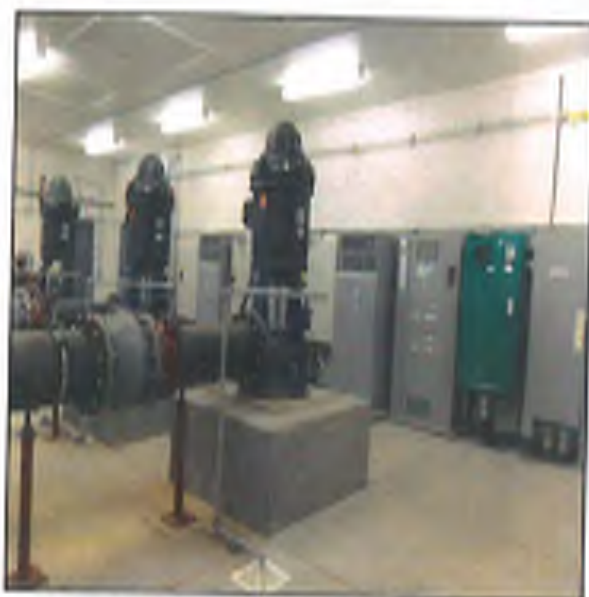
Fig. 30 - overall view of booster pumps and electrical panels
