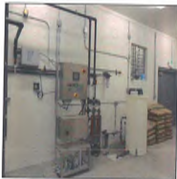
Fig. 31 - stand-by Miox treatment unit (not in use at time of survey)
