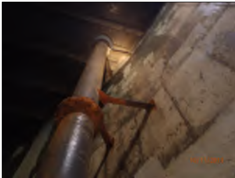
Overflow pipe and supports
