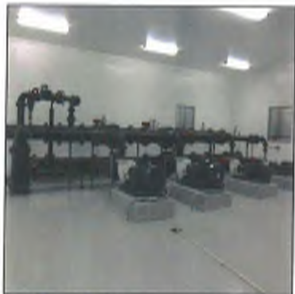
Fig. 61 – overall view of booster station associated with well # 9
