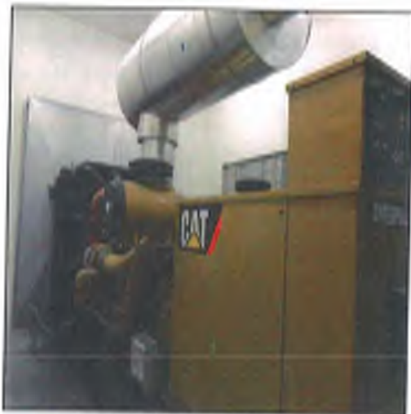
Fig. 55 – back-up generator within the booster station
