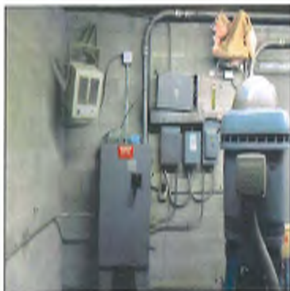
Fig. 5 – well # 5, electrical panel and heater
