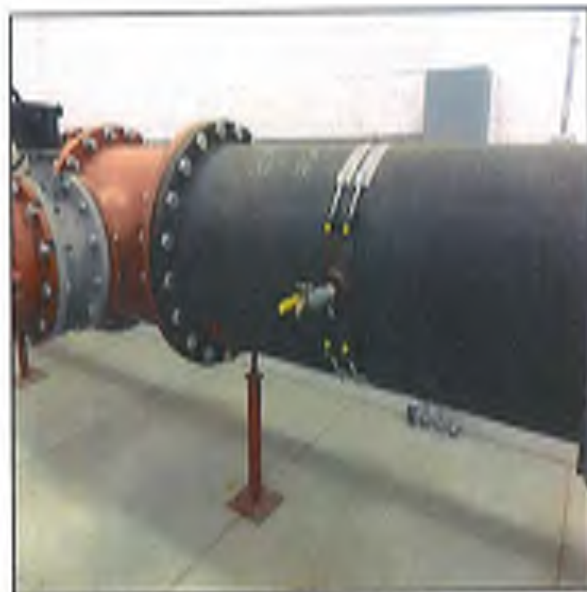
Fig. 27 – sample tap from 1.5 Million storage tank that is fed by well # 8
