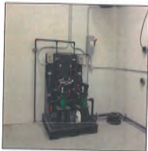
Fig. 32 - Miox unit - pumps
