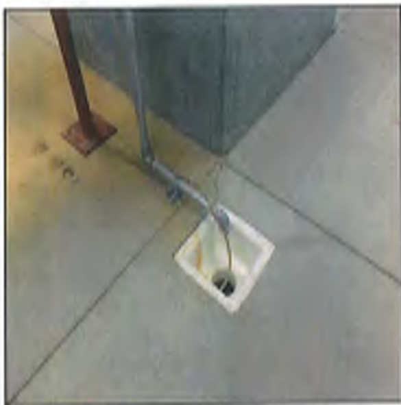
Fig. 25 – booster station floor drain
