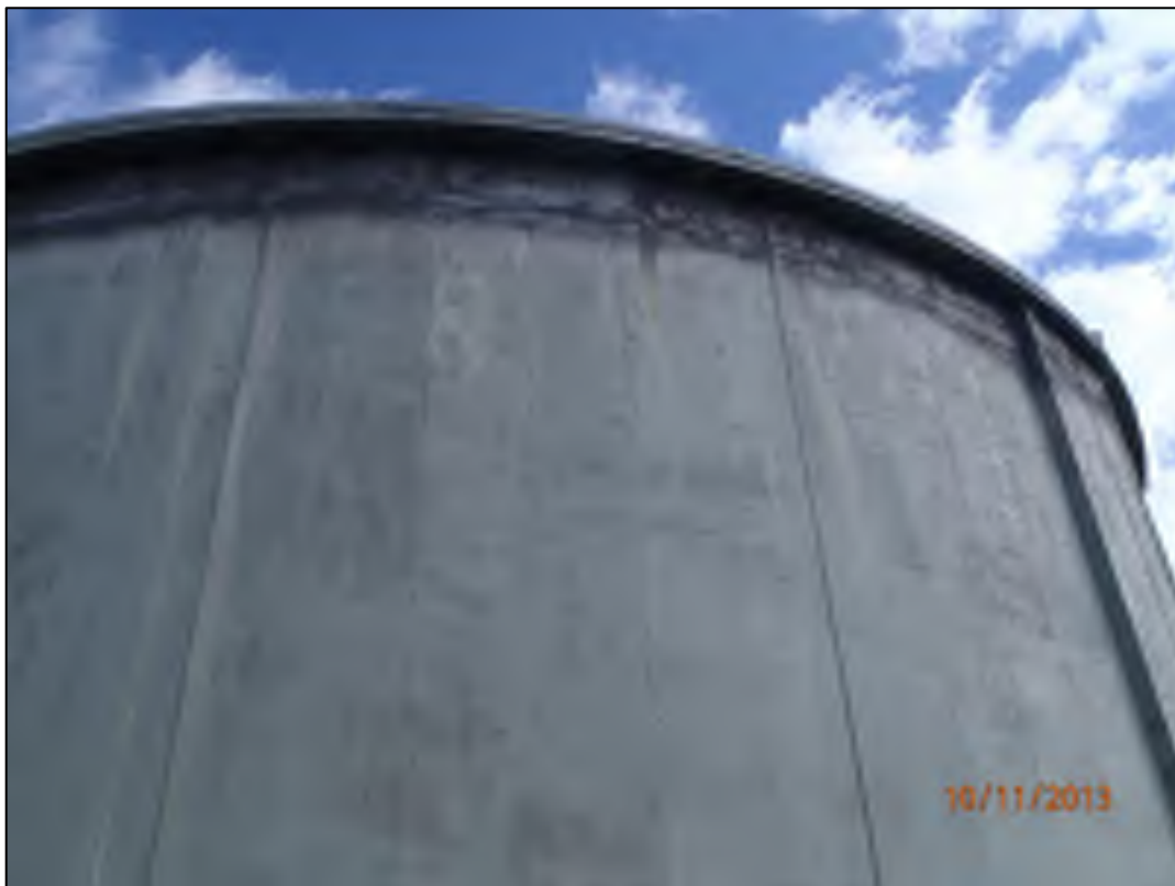
Patching at roof-to-wall joint experiencing moderate deterioration
