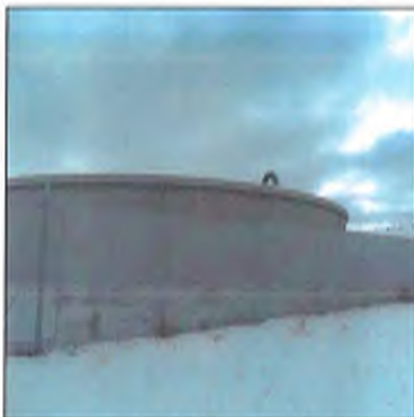
Fig. 15 – 1.5 Million/gal storage tank associated with well # 8 and booster station
