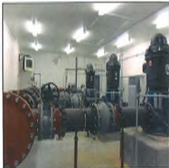
Fig. 26 – overall view of booster station
