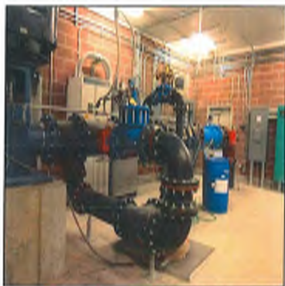
Fig. 66 – well # 11 discharge line (flow meter, check valve)
