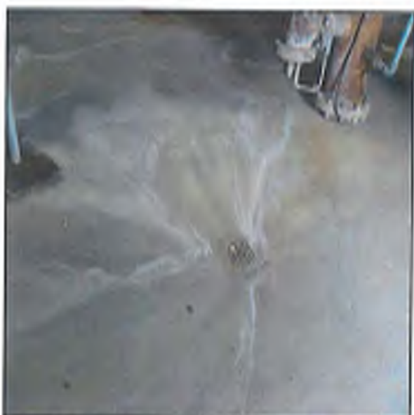
Fig. 12 – well house # 7 clean floor drain
