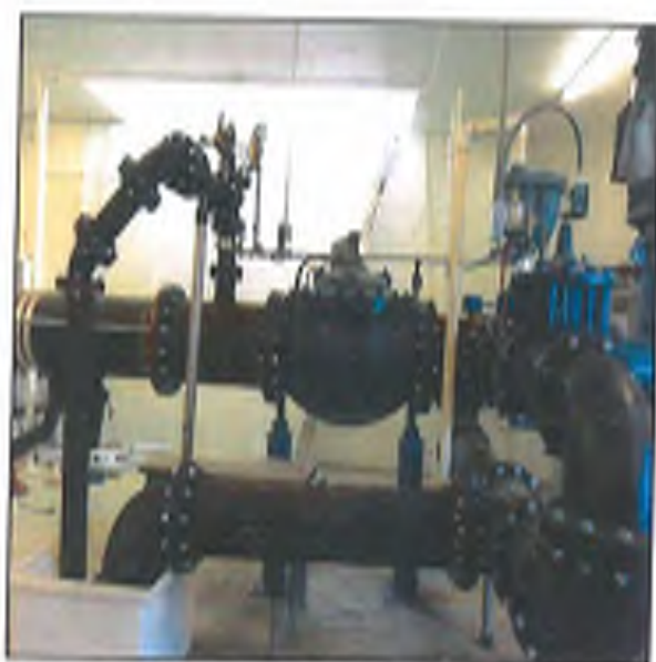
Fig. 45 - well # 10 discharge line
