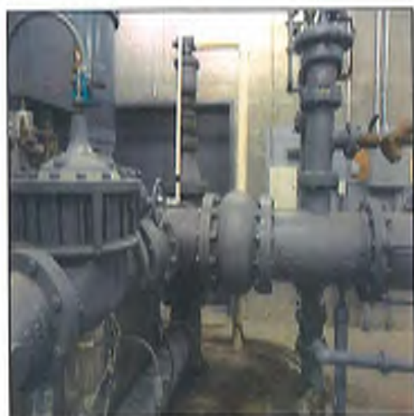
Fig. 20 – well # 8 check valve, pressure release and pressure
