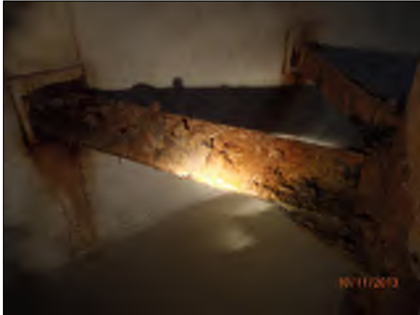
Close-up of rusting pipe supports
