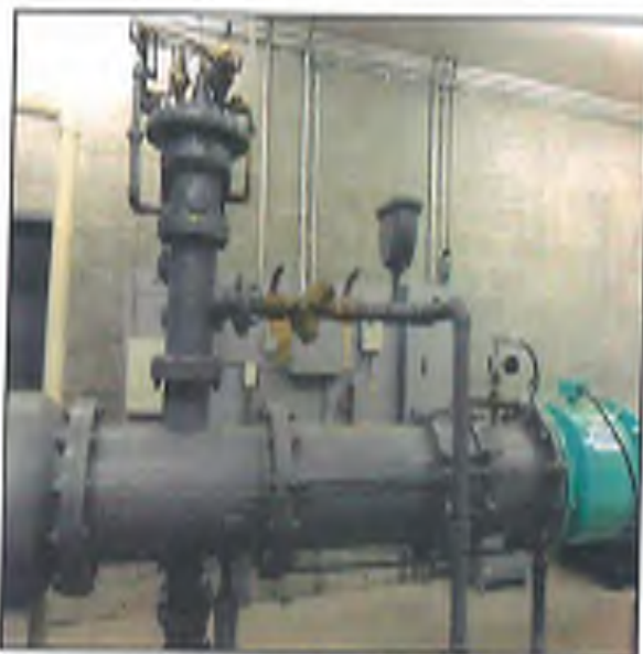
Fig. 21 – pressure reducer, double check valve, pressure relief, pressure gauge, source sample tap and flow meter on well # B discharge piping
