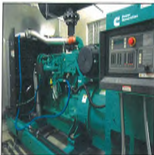
Fig. 33 – stand-by generator in booster station building
