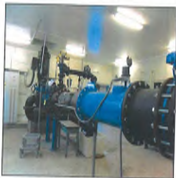
Fig. 46 - well # 10 flow meter and over view of discharge line
