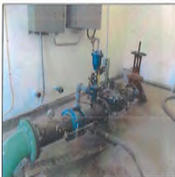
Fig. 39 – discharge piping from well # 2
