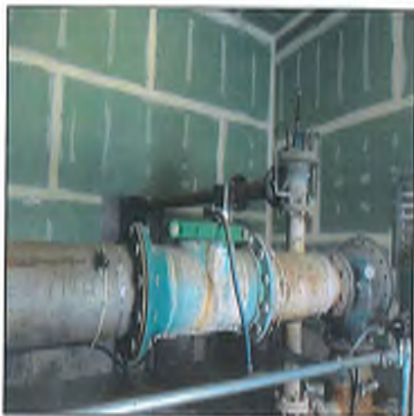
Fig. 10 – well # 7 flow meter
