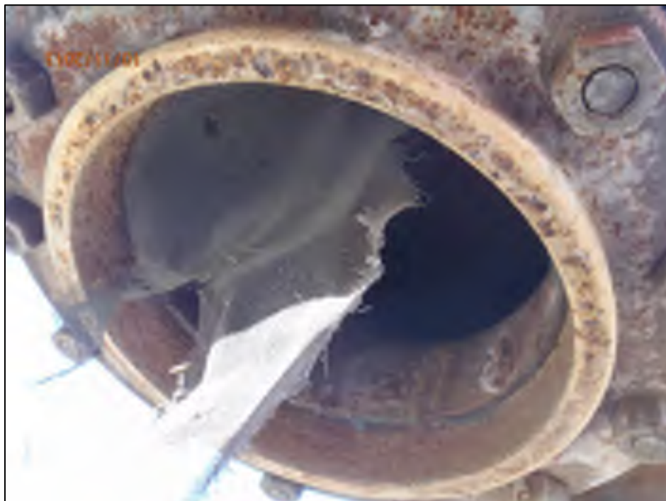
Overflow outflow mesh is damaged
