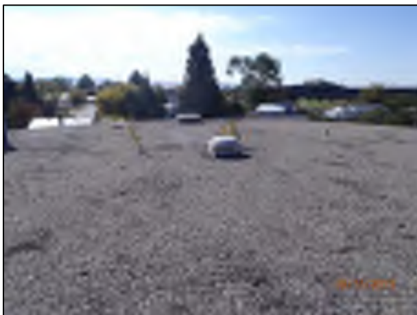
Tar and gravel roofing with tree growth
