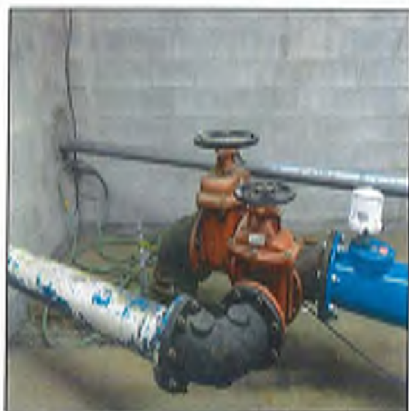
Fig. 3 – flow meter, isolation valves and pump to waste line
