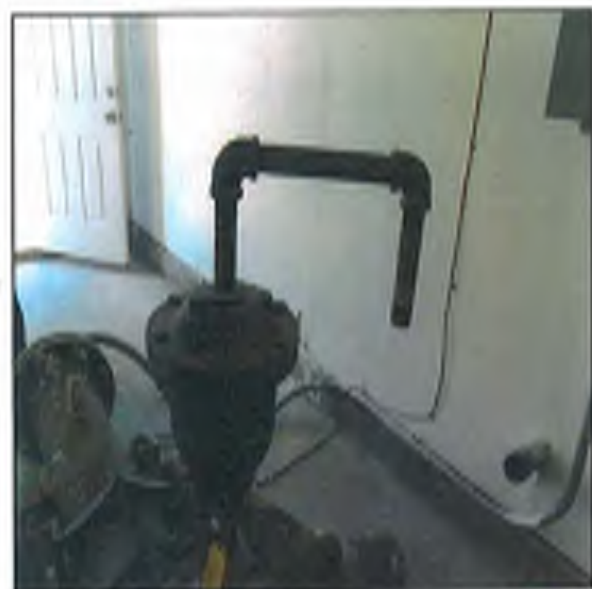
Fig. 41 – well # 2 unshielded air relief
