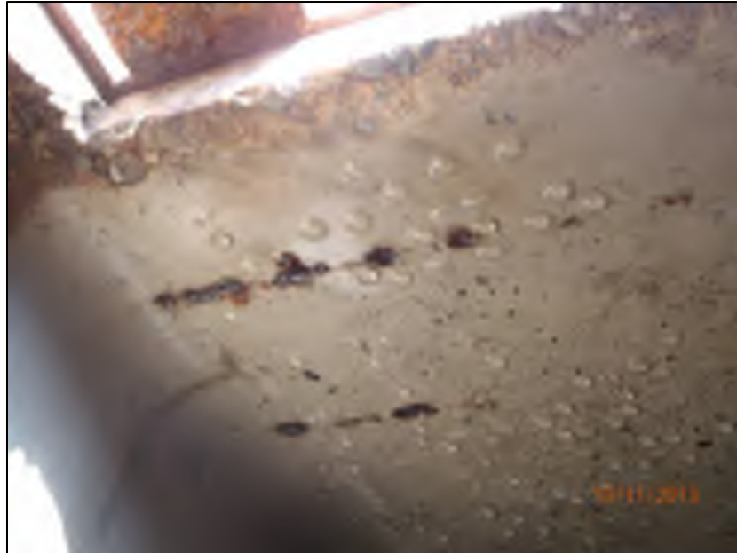
Rusting of reinforcing on underside of roof slab, lack of concrete cover
