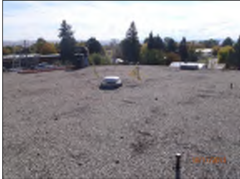
Roof access hatch and vent
