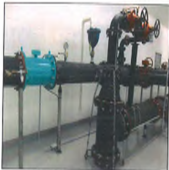
Fig. 62 – flow meter, pressure gauge, unscreened air release
