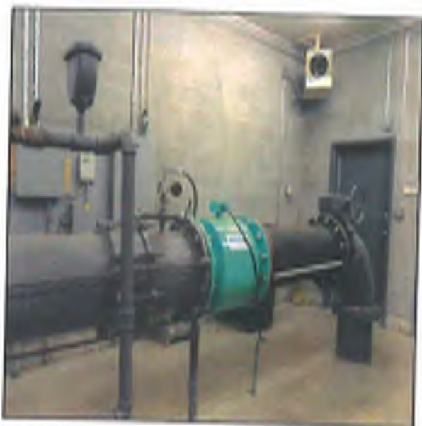
Fig. 22 – well # B discharge line and well house view
