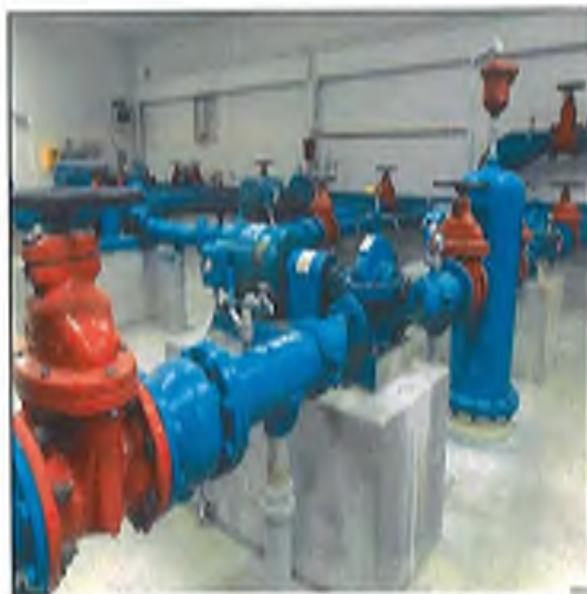
Fig. 52 – sample tap after storage tank
