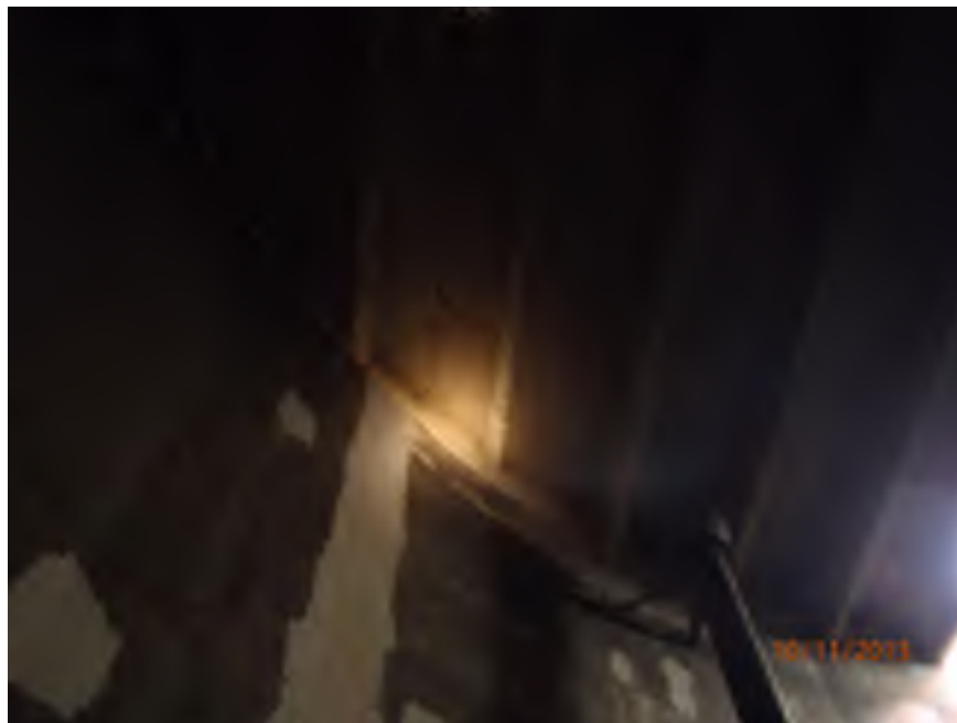
Cracking on underside of roof panel
