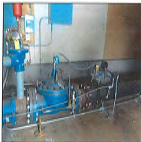
Fig. 35 – well # 3 check valve, pressure release and pressure reducer
