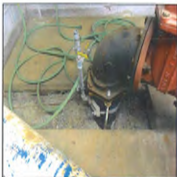
Fig. 6 – area used for potential drainage because well house # 5 lacks a floor drain
