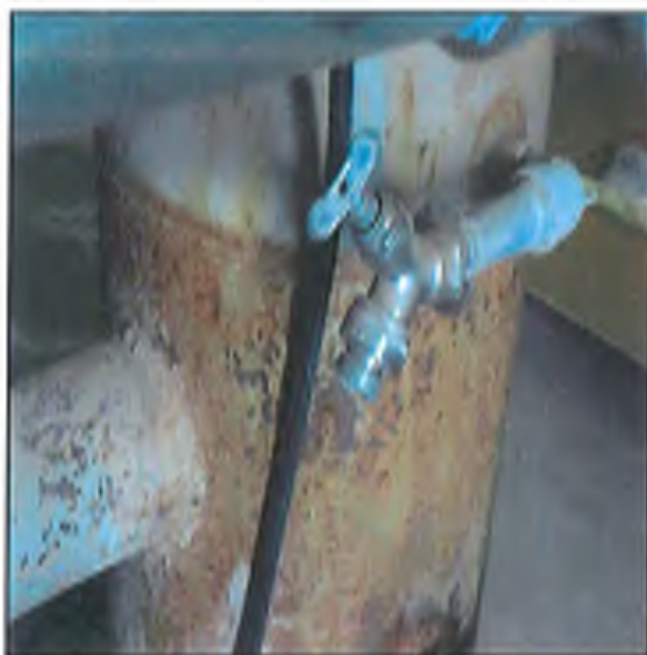
Fig. 11 – source sample tap equipped with a back flow device
