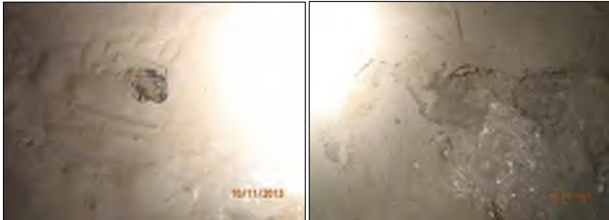
Boiling of coating removed; concrete appears to be in sound condition underneath
