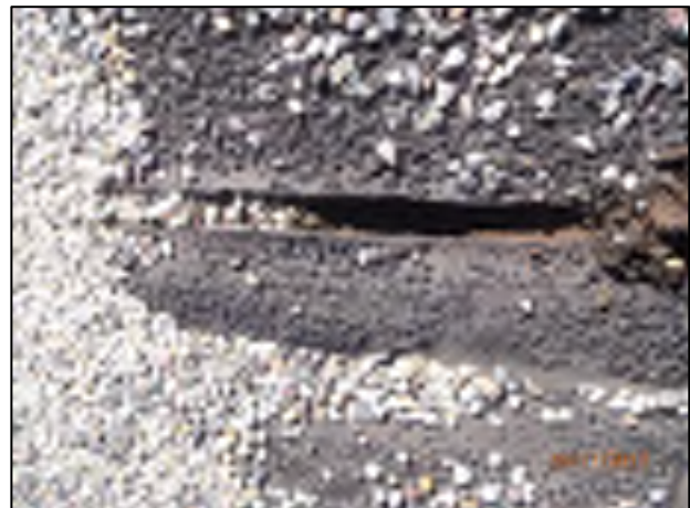
Peeling of roofing system
